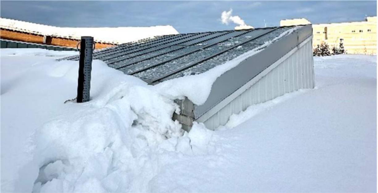
Image 4: Drifting Snow at Monoslope Skylight Feature (location #8).
