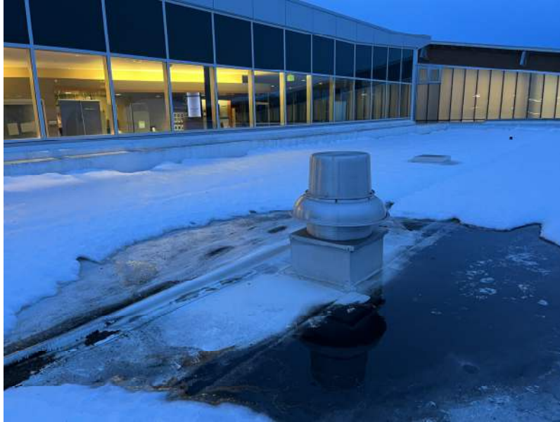
Figure 2: Sitting Water near Exhaust Fan
