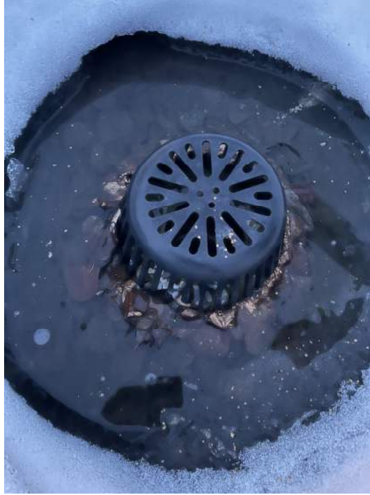
Figure 4: Drain Filled with Debris
