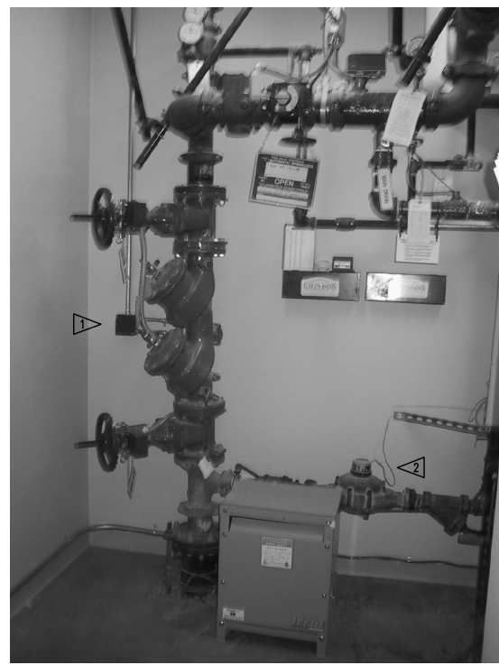
2 SPRINKLER RISER & CW SUPPLY MIS
